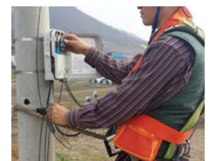
Work Belt on the telephone pole
